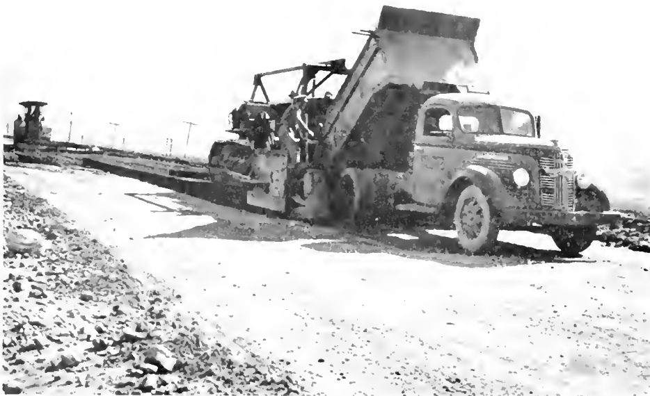
Spreading cement stabilized base. Note forward steel plate wing on bulldozer blade is mounted on wheel with screw jack adjustment
